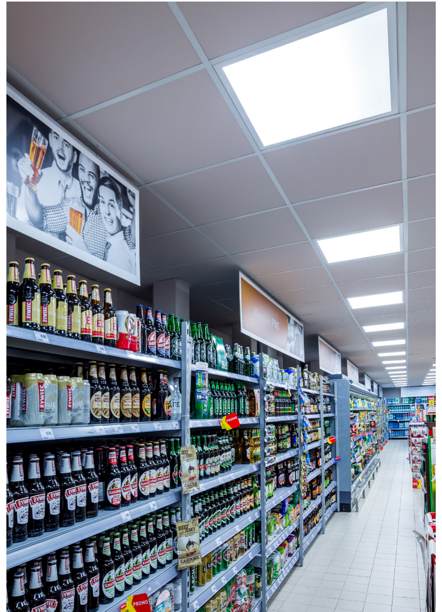
The use of the Plano LED Evo luminaire in the Intermarche store in Piekary Śląskie
