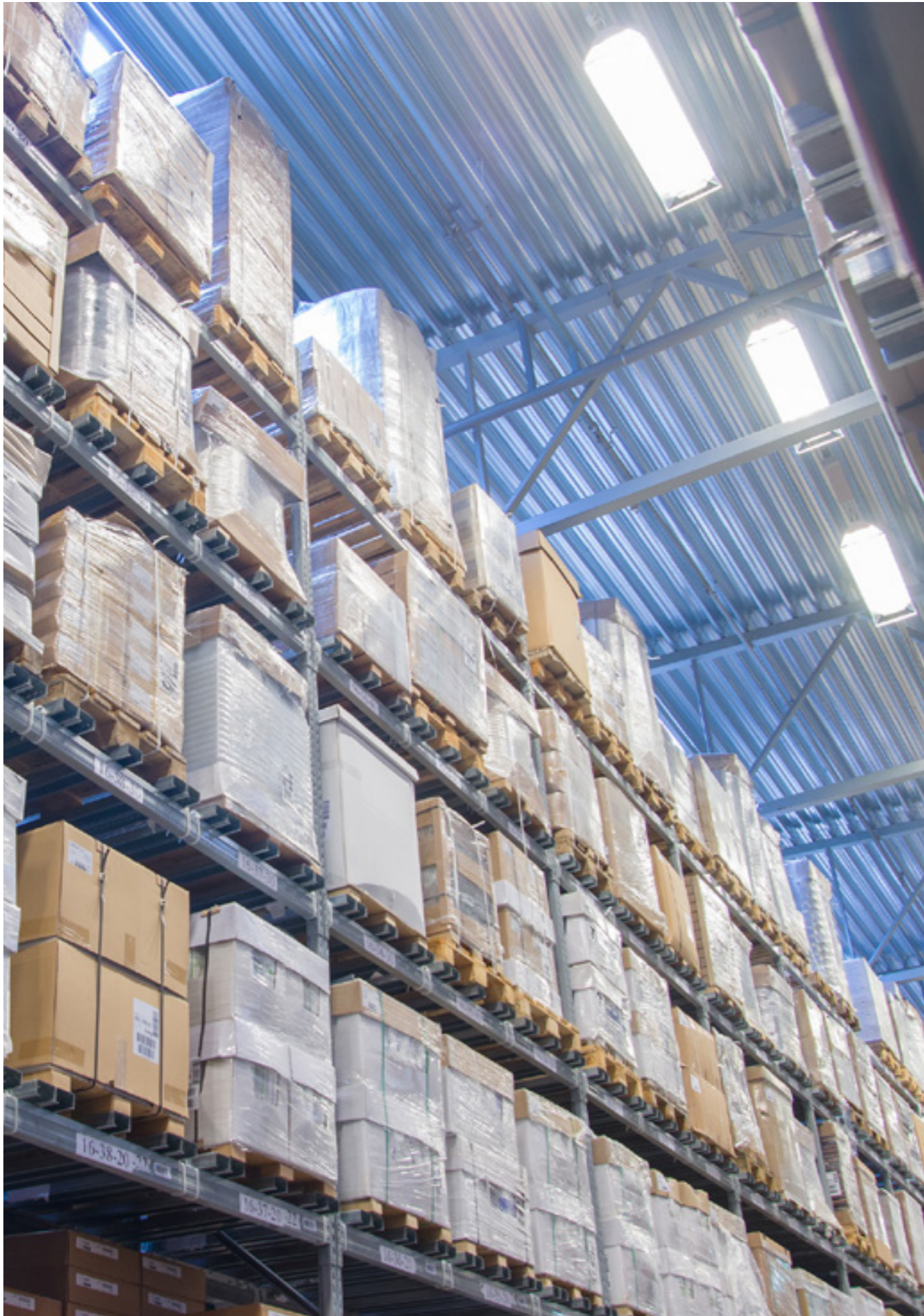
Application of the Industry 2 LED luminaire in a warehouse hall.
