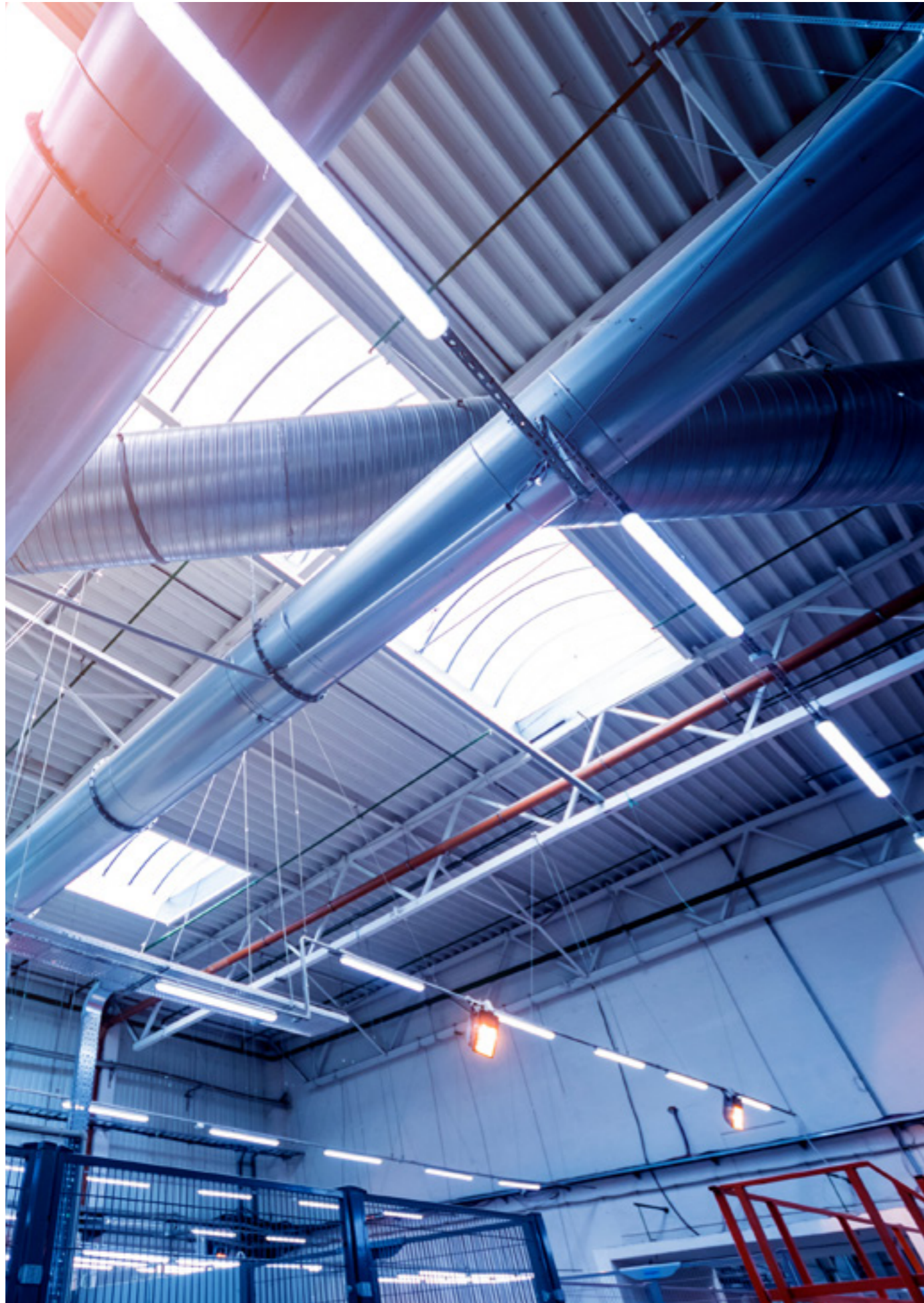
The use of Tytan 2 LED Endura luminaires in a warehouse hall
